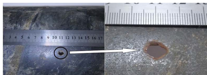
Figure 1: The external surface of the 8-inch pipe, the pipe was perforated due to internal corrosion.
